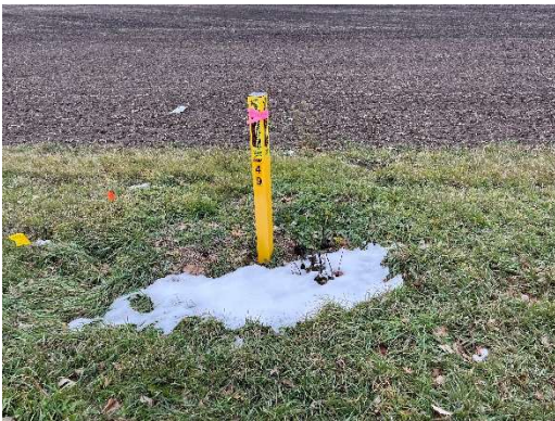
View of Petroleum Pipeline Near the Northeast Corner of 02-19-200-006
